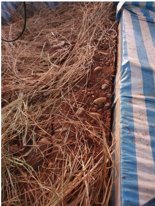
(c)坡頂張力裂縫
