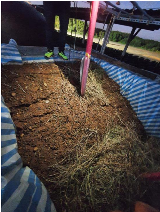
(a)坡面張力裂縫
