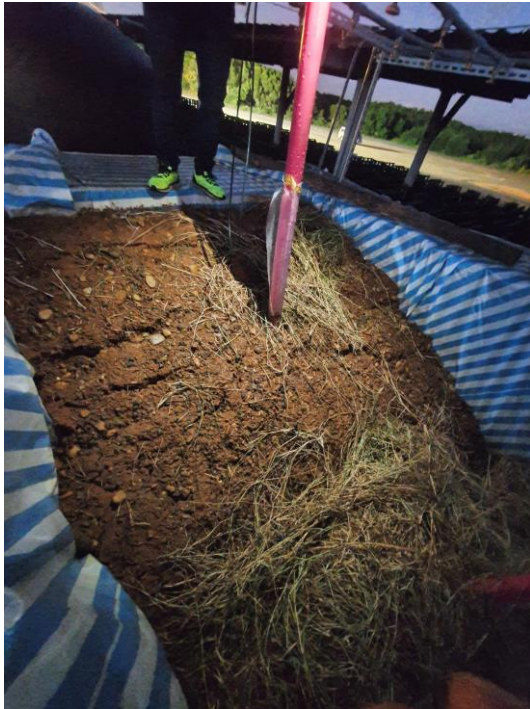
(a)坡面張力裂縫
