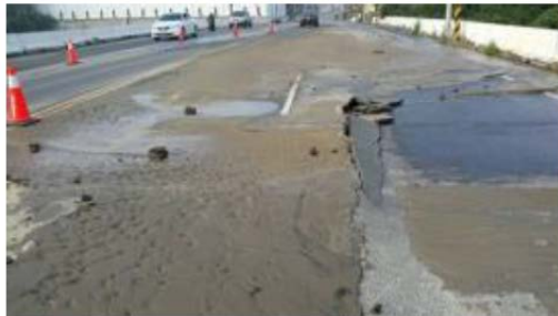
(a)開運橋頭(永康側)破管
