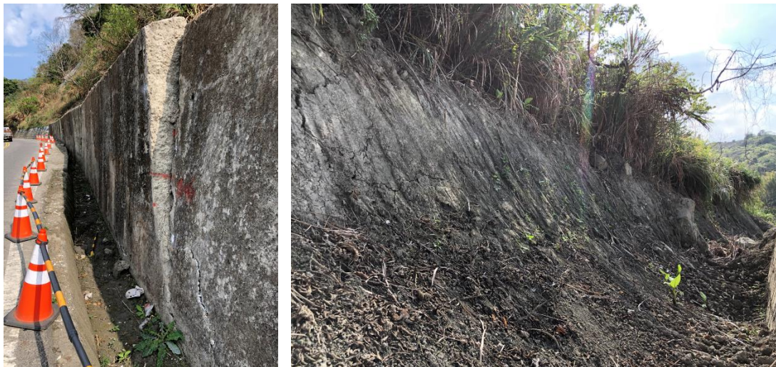
(a) 擋土牆傾倒
