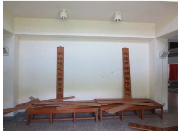
(b)隔間牆損壞
