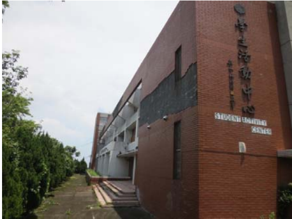
(a)外牆磁磚掉落
