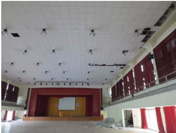
(c)天花板損壞
